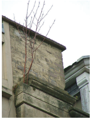
Vegetation growing out of City Centre property—roots of plants and trees cause opening of mortar joints and can lead to damp problems and unstable stonework.
